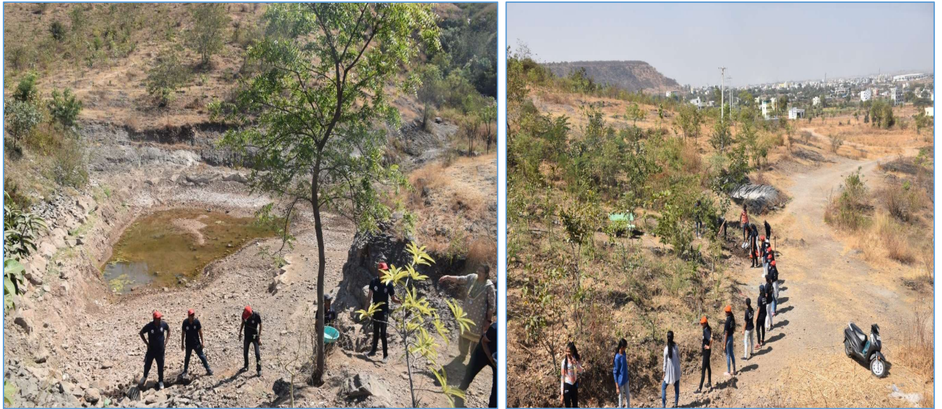
Farm Pond renovation for upcoming rainy season tree plantation in Bakori Forest Project.
